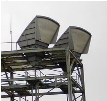
C band horn-reflector antennas on the roof of a telephone switching center
